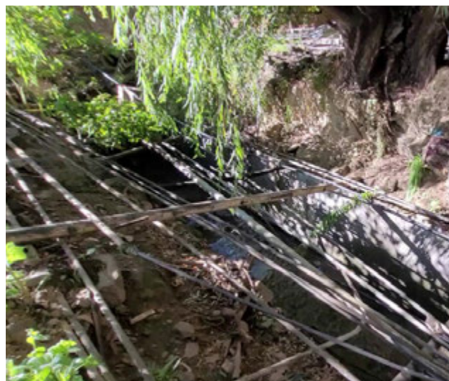
Figure 6.55 Concrete Channel - Unmaintained and Multiple Utilities
