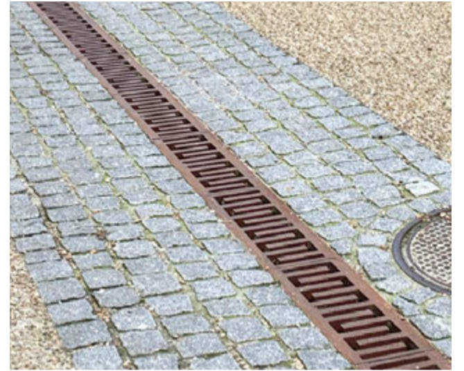
Figure 4.71 Introducing water safely within a confined space - the decorative grill means that the sound of running water will be apparent, while reducing trip hazards.
