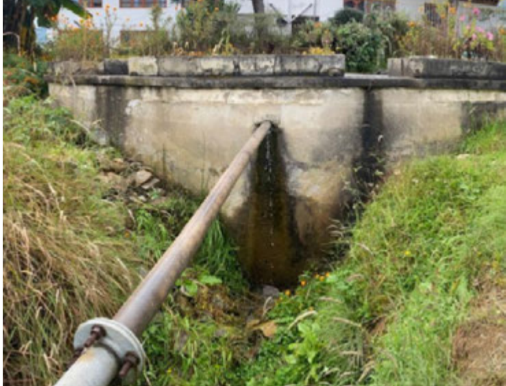
Figure 6.53 BCCI Tank Overflowing (From Water Loss Audit)
