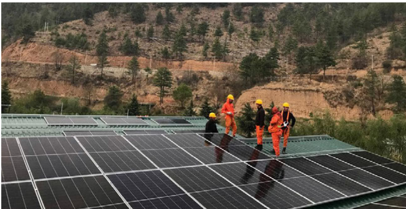
Figure 3.111 CFM rooftop solar plant.
