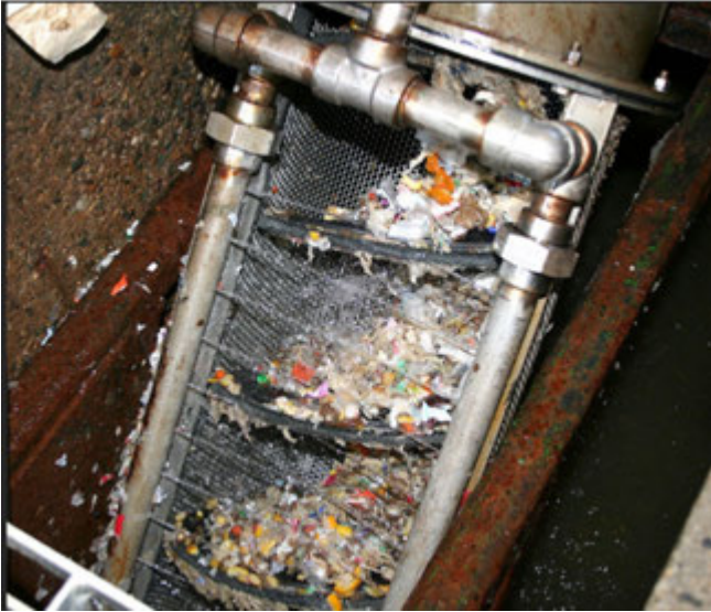
Figure 5-18: Example Wastewater Screen (Source: JWC Environmental)
